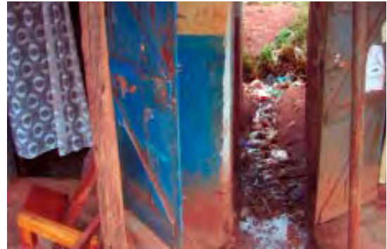
Poor drainage. Photo: © Kampala city council
