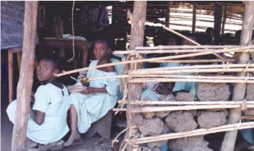
Uganda: collapsing classroom walls at Kanyunyu Primary School
